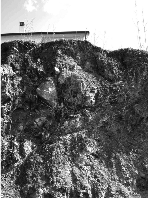
Fig. 3 - Photograph showing a road scarp in the Seluci di Lauria.
