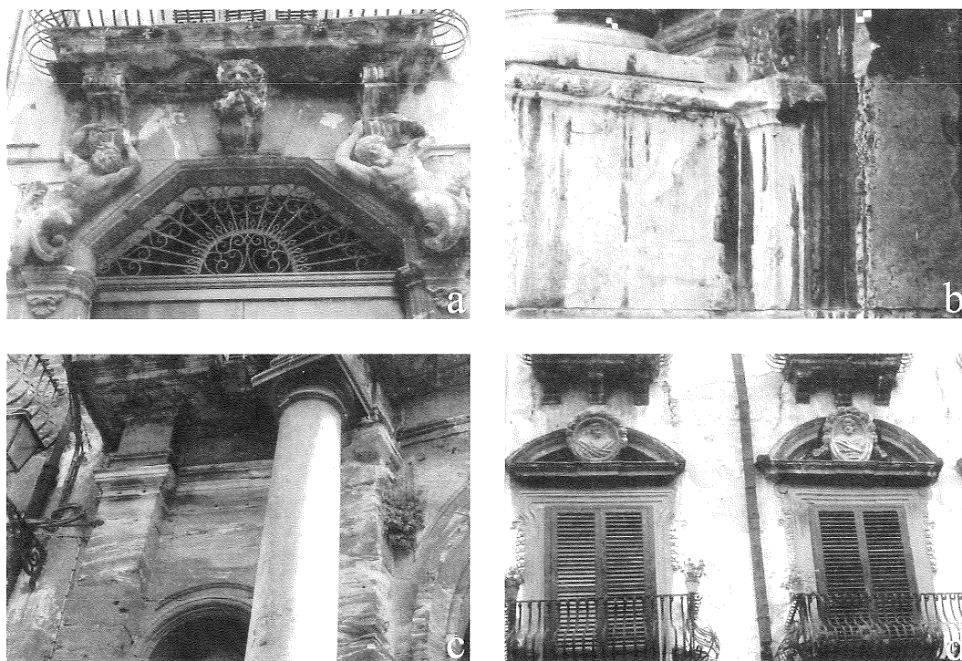
Fig. 2 – (a) Ugo delle Favare palace (XVII century): soluble salt efflorescences and black crusts; (b) Alliata di Villafranca palace (XVIII century) brownish-black films on Billiemi limestone; (c) Alliata di Villafranca palace (XVIII century) examples of black crusts and differential degradation in the biocalcarenite; (d) Lungarini Palace: detachment of the XVIII century plaster bringing to light the older one (XVII century) decorated with a painted «diamond» ashlar-work.
